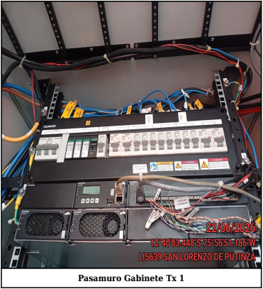
Pasamuro Gabinete Tx 1
