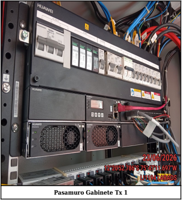
Pasamuro Gabinete Tx 1
