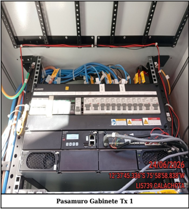
Pasamuro Gabinete Tx 1
