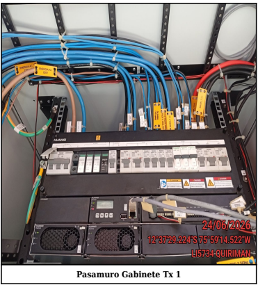
Pasamuro Gabinete Tx 1
