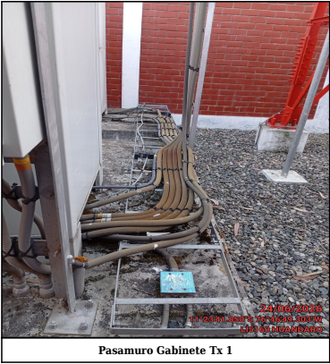
Pasamuro Gabinete Tx 1
