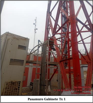
Pasamuro Gabinete Tx 1
