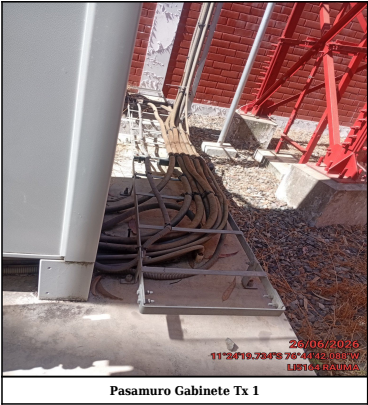
Pasamuro Gabinete Tx 1
