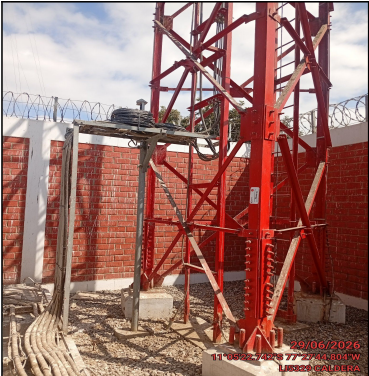
Pasamuro Gabinete Tx 1
