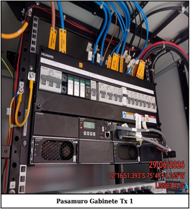
Pasamuro Gabinete Tx 1
