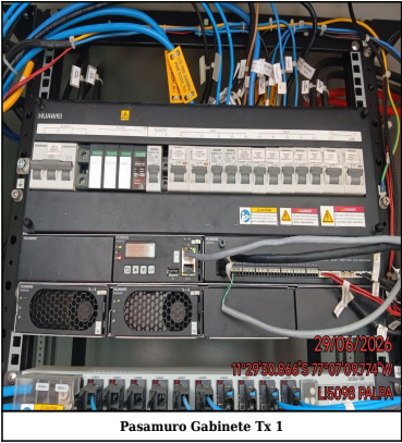
Pasamuro Gabinete Tx 1
