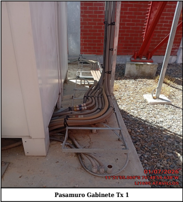
Pasamuro Gabinete Tx 1
