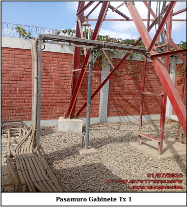
Pasamuro Gabinete Tx 1
