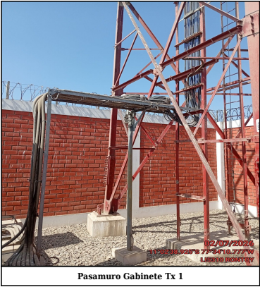
Pasamuro Gabinete Tx 1
