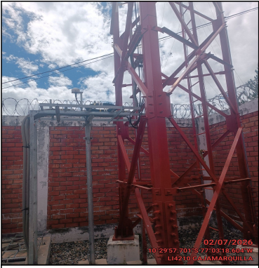
Pasamuro Gabinete Tx 1
