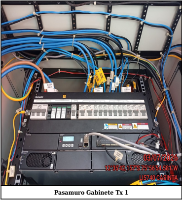
Pasamuro Gabinete Tx 1
