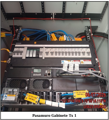
Pasamuro Gabinete Tx 1
