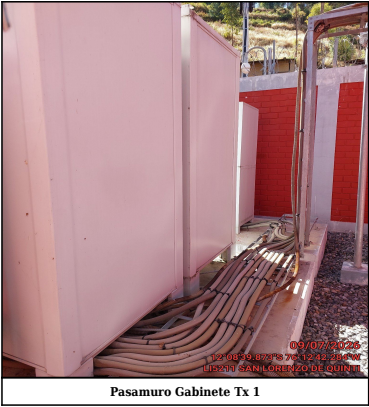
Pasamuro Gabinete Tx 1
