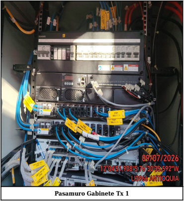
Pasamuro Gabinete Tx 1
