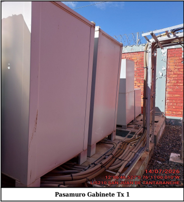
Pasamuro Gabinete Tx 1
