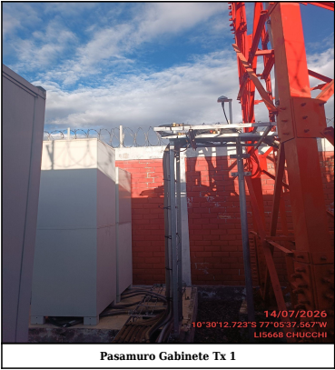
Pasamuro Gabinete Tx 1
