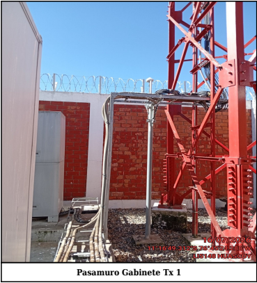
Pasamuro Gabinete Tx 1
