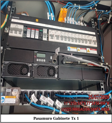
Pasamuro Gabinete Tx 1
