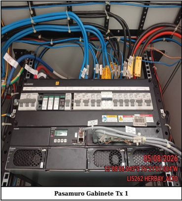
Pasamuro Gabinete Tx 1
