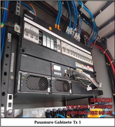
Pasamuro Gabinete Tx 1
