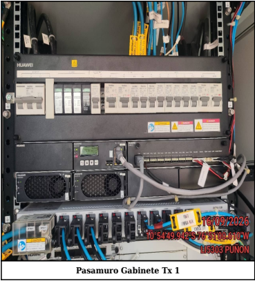
Pasamuro Gabinete Tx 1
